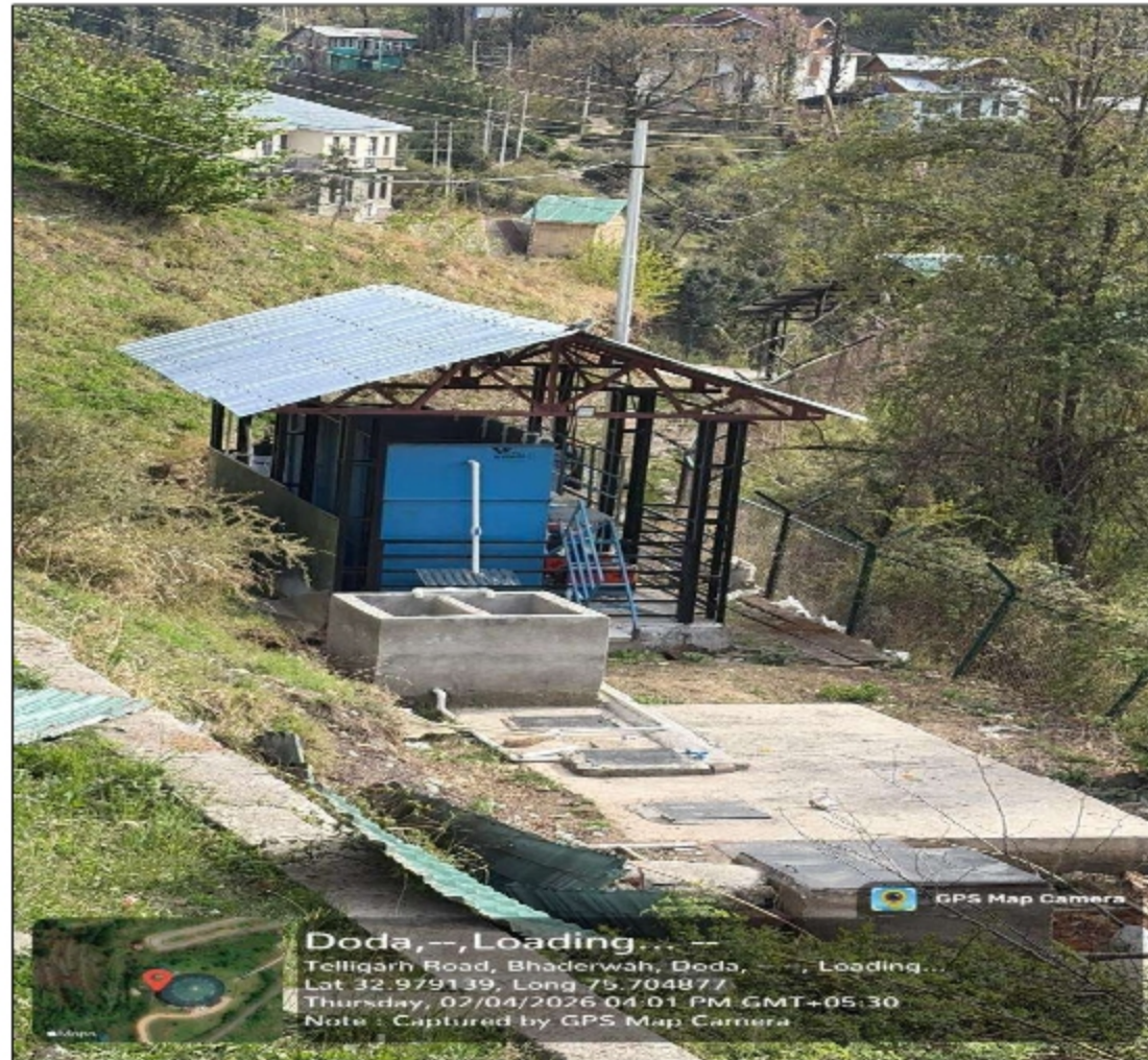
STP installed at Teligarh Resort, Bhaderwah
